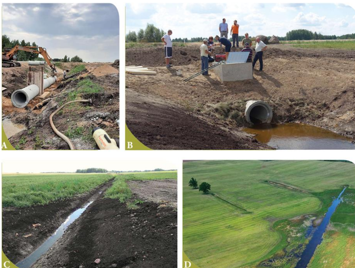
Reconstruction of a drainage system in Baisogala site and its surroundings, in 2022: A–B – installation of a sluice regulator with a water outlet (© UAB Baisogalos statyba, Jūratė Sendžikaitė), C – cleaned and reshaped drainage ditch (© Jūratė Sendžikaitė), D – restructured and resurfaced drainage headers (left) and dammed drainage ditch (right). © Nerijus Zableckis
